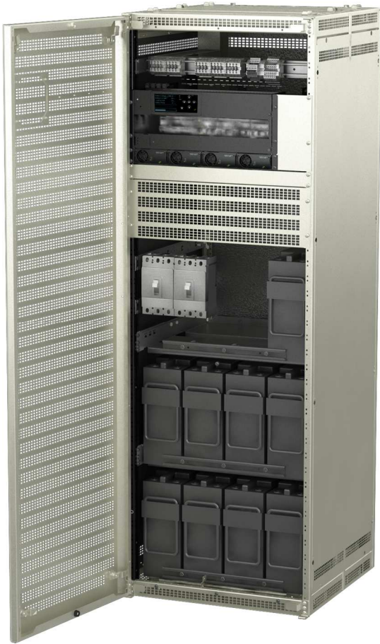
IBB SYSTEM IN FPC CABINET
